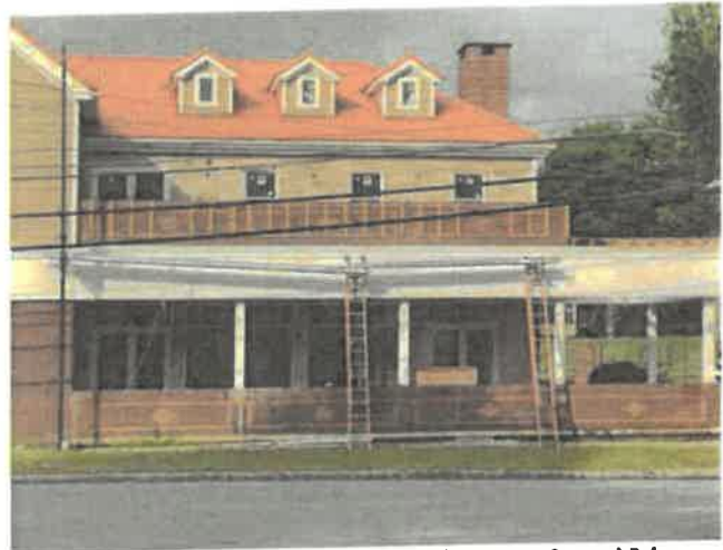
Non-Conforming Brick Siding and Railing on 2 nd Floor Deck. Billboard Interpretation of Doric or Tuscan Order in Non-Conformance with Approved Design Features.
