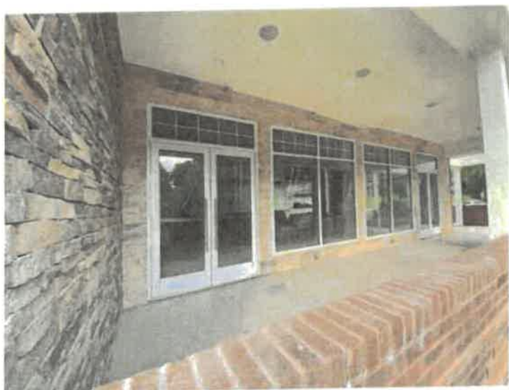
Travertine and Cultured Stone Siding in Non-Conformance With Approved Defining Features.
