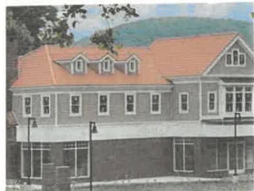
Synthetic Faux Spanish Barrel Tile Roof in non-conformance with Approved Design Features. Non-Approved Brick.
